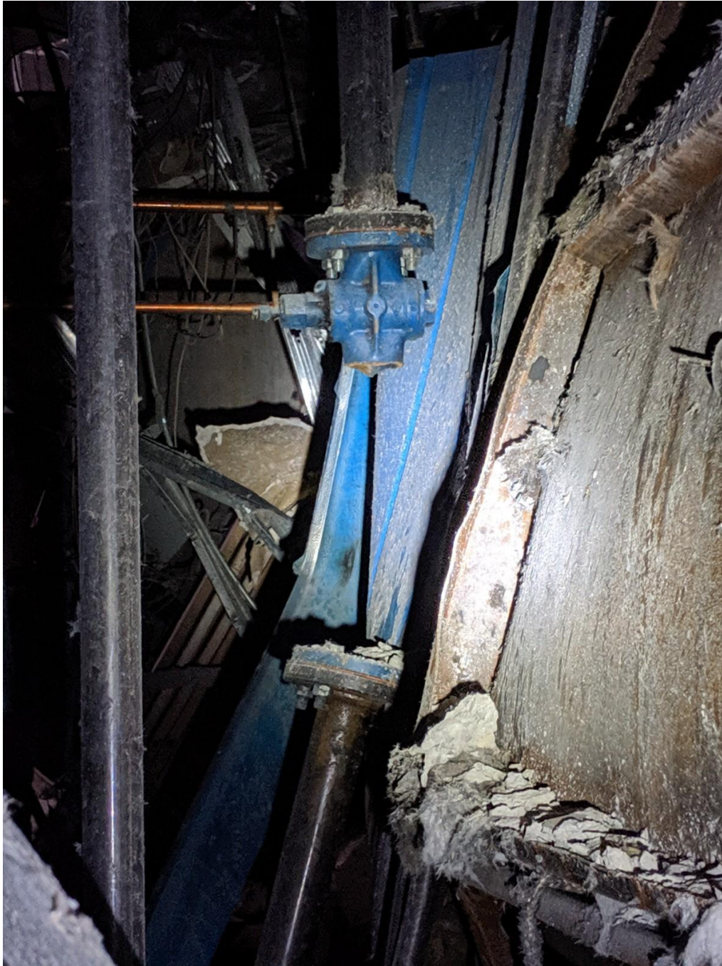
Figure 4. A view of the primary gas shut-off valve on Boiler #1 exhibiting damage from the initial explosion.
