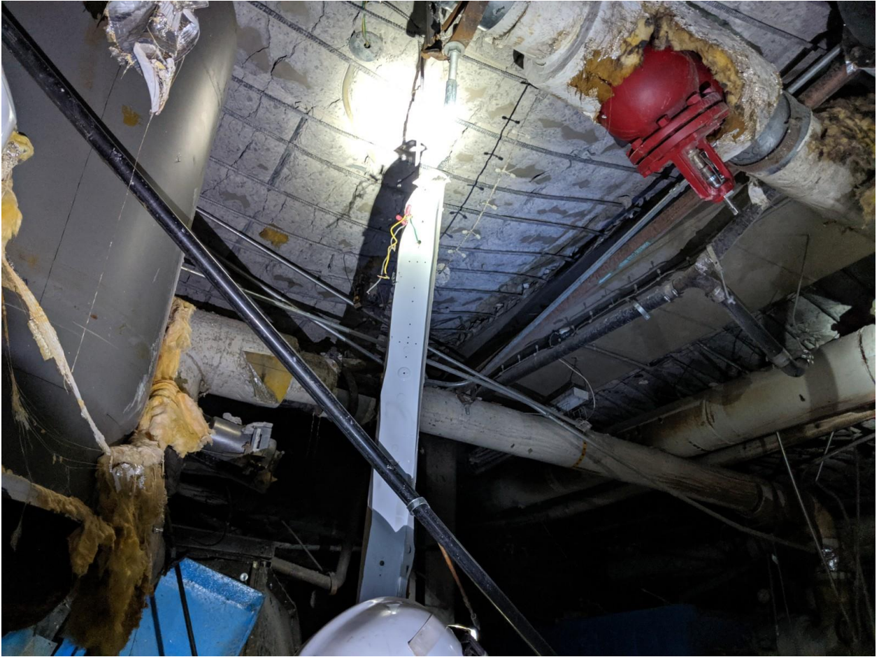
Figure 6. Ceiling of the boiler room. Damage is consistent with a significant blast pressure wave caused by a gas explosion.
