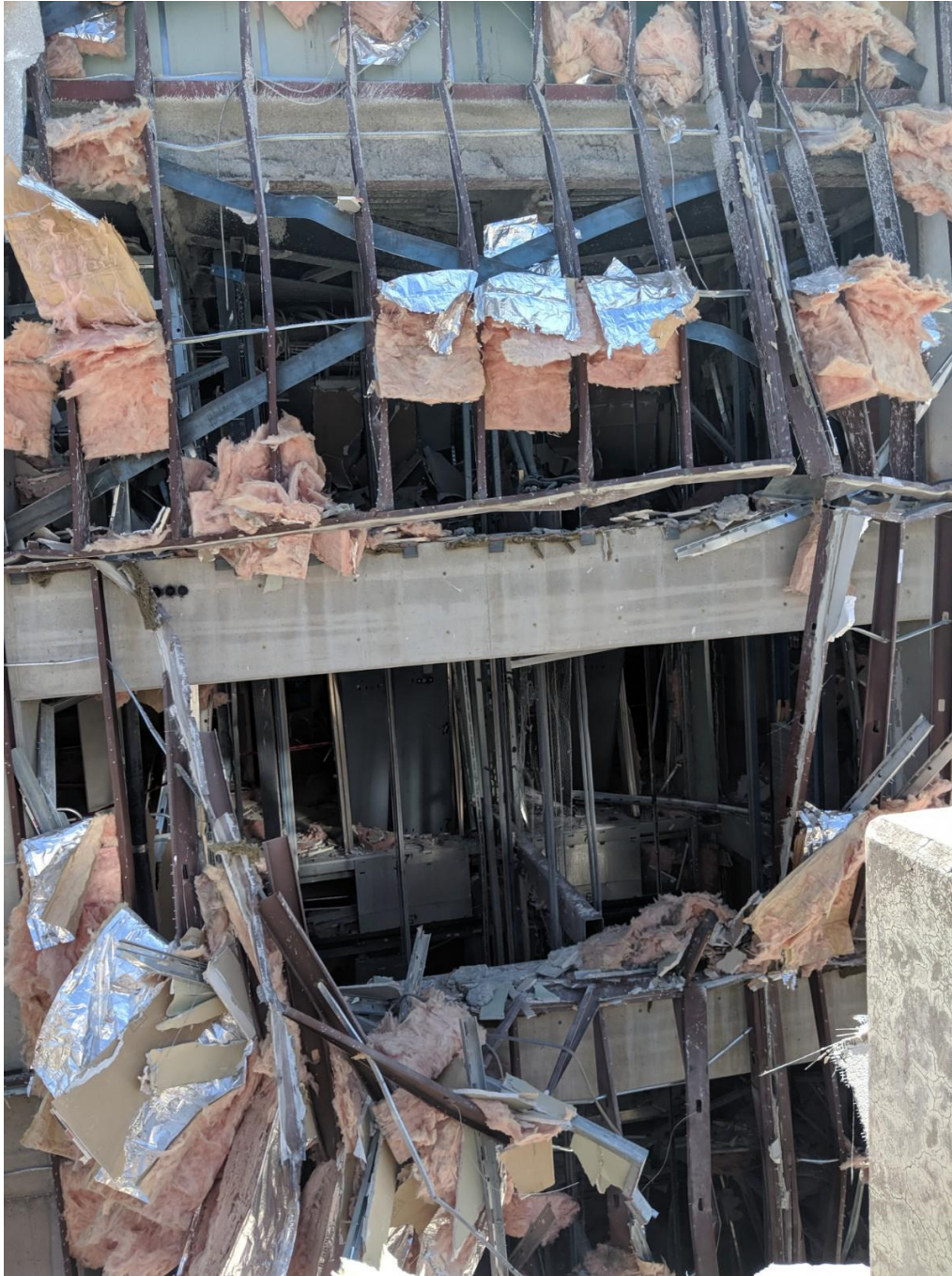
Figure 5. Argenta Hall elevator hoistway, as seen from the roof of Nye Hall. Damage is consistent with a significant blast pressure wave caused by a gas explosion.
