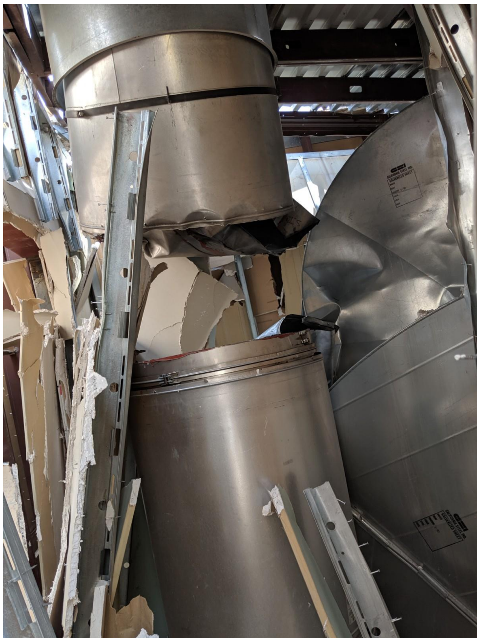
Figure 3. Exhaust assembly from Boiler #1. This is the view inside of the ducting area on the roof of Argenta Hall. Damage is consistent with an explosion occurring within this assembly.
