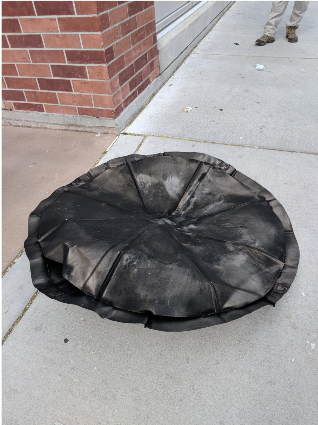
Figure 2. Rain shield from Boiler #1 exhaust assembly, found on the North side of Nye Hall. Damage is consistent with an explosion within the exhaust assembly.
