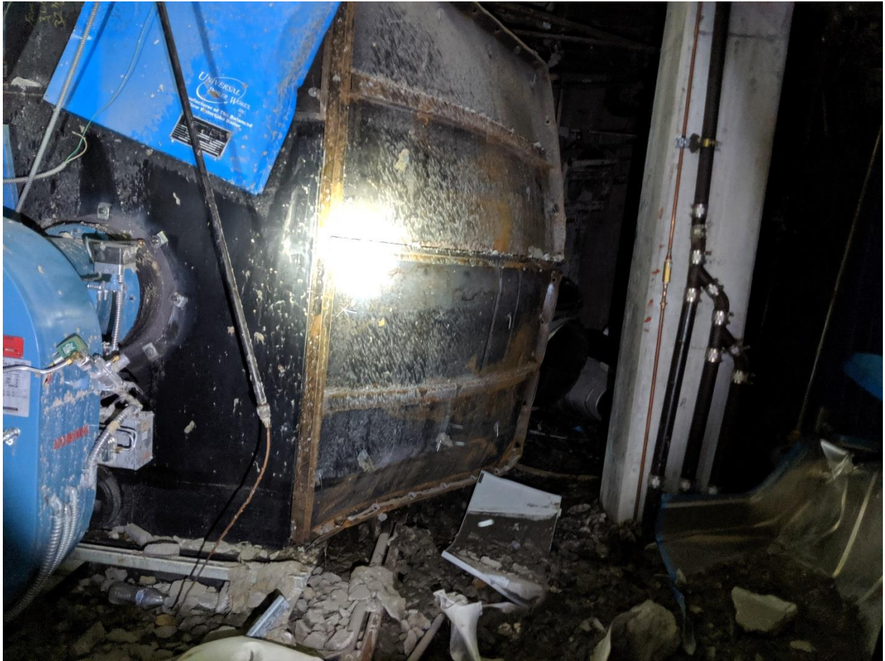
Figure 1. A front view of Boiler #1, showing damage from internal explosion of the furnace assembly.
